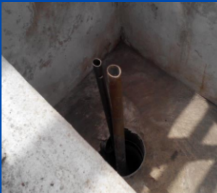
Revamped deepwell groundbed for NPDC/ Heritage Energy Operational Services Warri, Delta State Operator of OML 30
