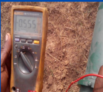
Pipe to Soil Potential measurement at the unprotected side of the insulating joints of flow lines for NPDC/Heritage at Ewreni Flow station
