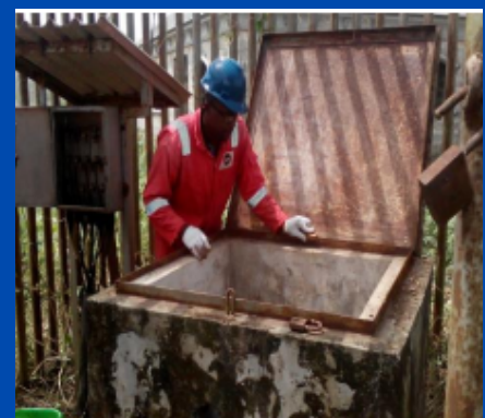
Cleaning and maintenance of anode deepwell ground for Heritage/NPDC at Evwreni Flow station
