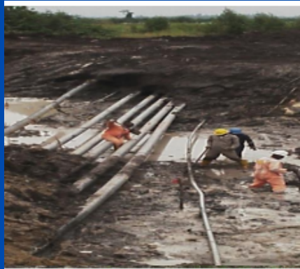
Installation of Cathodic Protection system on various flow lines at Soku Flow Station
