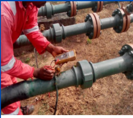
Pipe to Soil Potential measurement at the insulating joints of flow lines for NPDC/Heritage at Oroni Flow station
