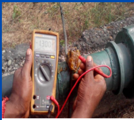
Pipe to Soil Potential measurement at the protected side of the insulating joints of flow lines for NPDC/Heritage at Kokori Flow station
