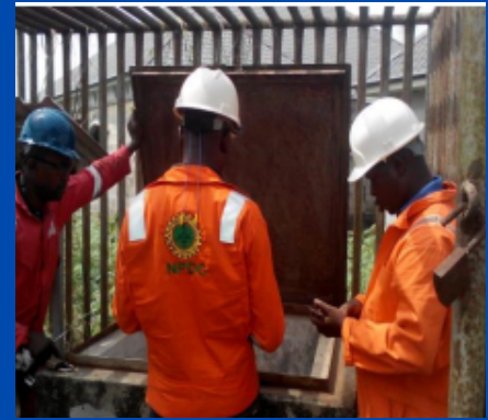
Inspection of upgraded and revamped deepwell groundbed by a combined team of NPDC/Heritage and Princcatar Imperial Nig. Ltd.
