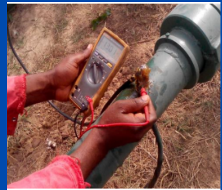
Pipe to Soil Potential measurement at the insulating joints of flow lines for NPDC/Heritage at Ewreni Flow station on several flow lines at Soku Flow Station
