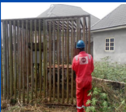
Well-head security pit housing the groundbed and 8-way positive junction box for Heritage/NPDC flow station at Oroni
