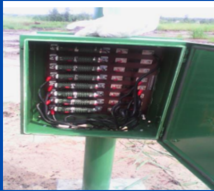
Junction box for cathodic protection interference mitigation for pipe crossings at Ebelle OKpekpe for BUA Edo Cement Factory 16'' x 22km Pipeline project
