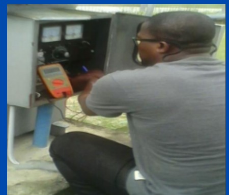
Installation of Air cooled transformer rectifier unit at NLNG Bonny for Akiama-Finima Water borehole project
