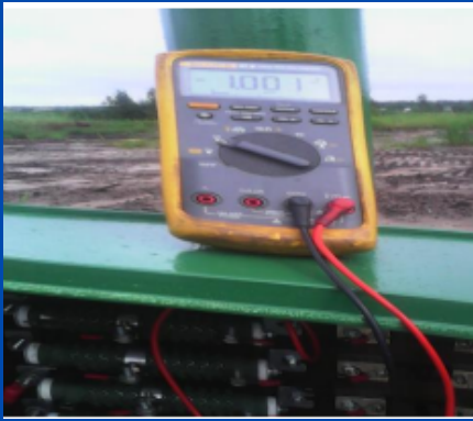
Pipe to Soil Potential Measurement of installed Interference mitigation junction box Ebelle OKpekpe for BUA Edo Cement Factory 16'' x 22km Pipeline project
