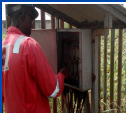
Trouble shooting, repairs and maintenance on positive junction box for Heritage/NPDC OML 30 Kokori Flow station
