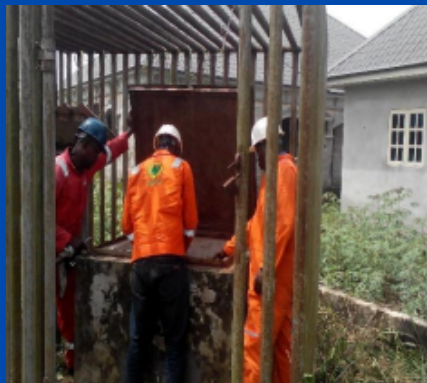
Inspection of upgraded and revamped deepwell groundbed by a a combined team of NPDC/Heritage and Princcatar Imperial Nig. Ltd
