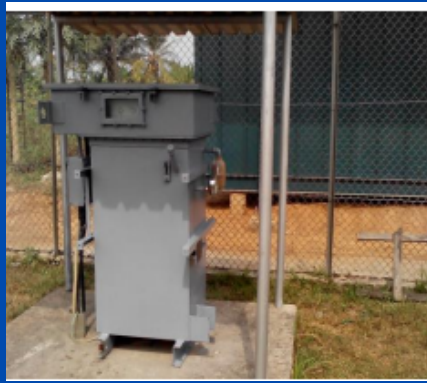
Installed Transformer Rectifier at Oroni Flow station for NPDC/Heritage Energy Operational Services Warri, Delta State operator of OML 30
