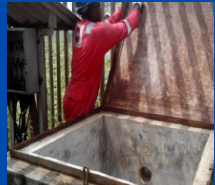
Cleaning and maintenance of anode deepwell ground for Heritage/NPDC at Evwreni Flow station
